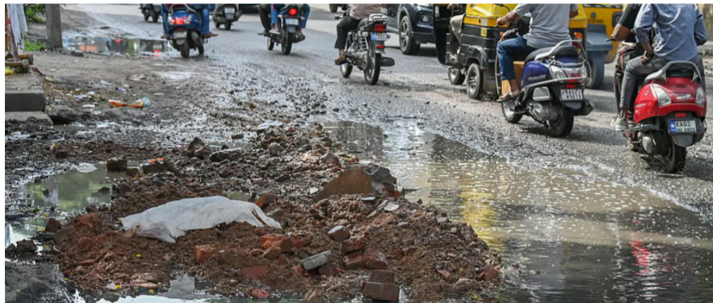
Potholes and debris on Hombegowda Nagar main road
