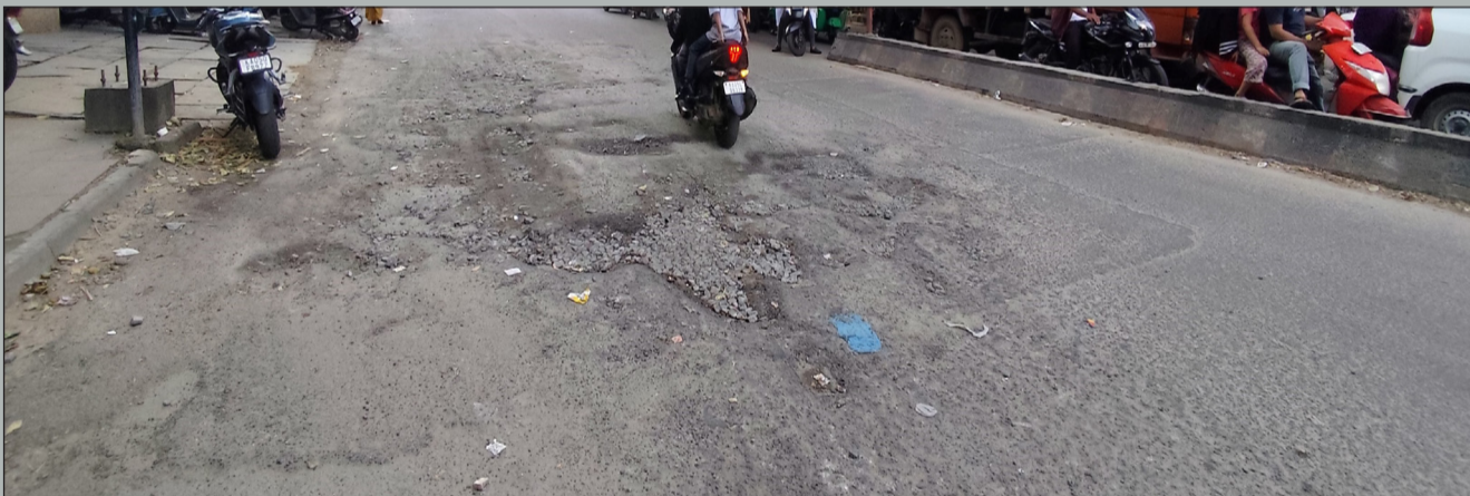
Tilak Nagar main road with unrepaired potholes
